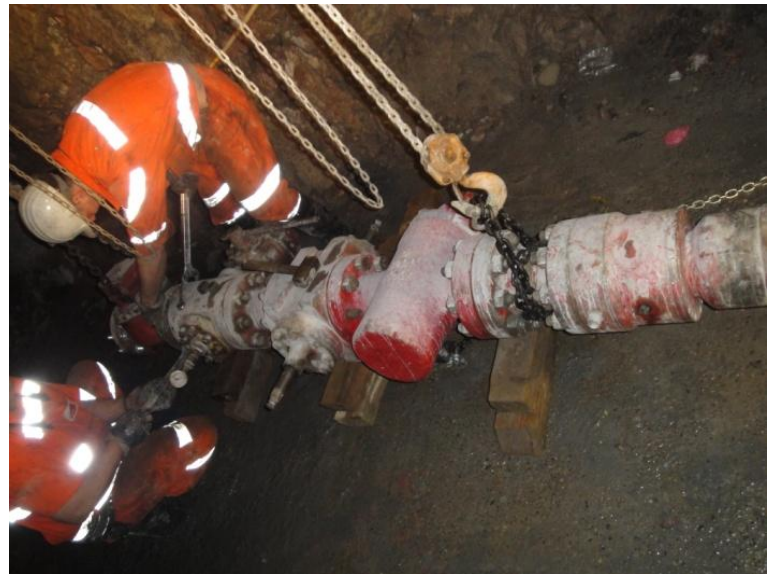
Figure 2: Fitting the preventer system
